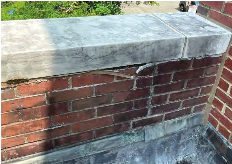
Deteriorated sealant resulting from adhesion failure and inappropriate placement of sealant at a coping bed joint, where water became trapped in the adjacent mortar and caused freeze/thaw damage and biological growth.
