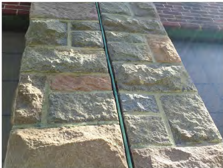
Vertical copper sheet metal expansion joint in a historic stone masonry wall.
