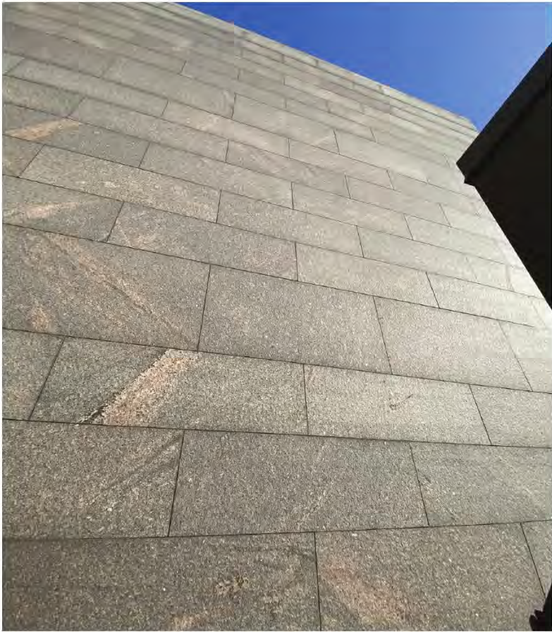
Stone masonry joints with recessed rigid foam pad infill in a mid-century modernist style building.
