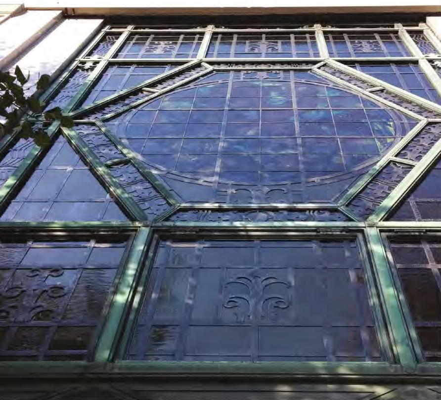
Historic stained-glass window with fully restored lead came and linseed oil joints between glazing panes.
