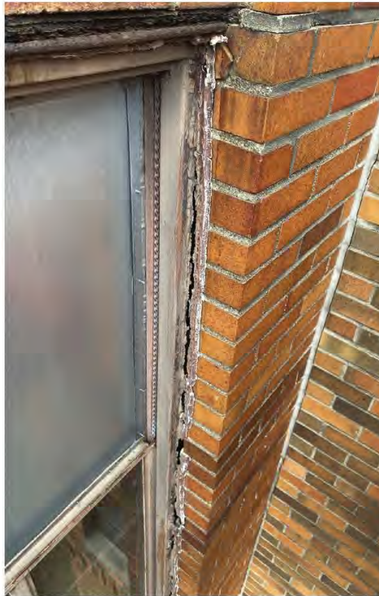
Deteriorated sealant at metal window perimeter resulting from cohesion failure and a lack of backer material, and also from age and ultraviolet (UV) exposure, making the material dry and brittle. Also note open vertical mortar joint at masonry corner exhibiting adhesion failure from building movement.
