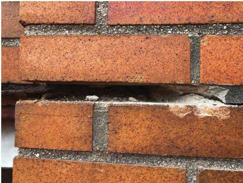
Deteriorated and open mortar joint in a brick masonry wall resulting from jacking of the adjacent corroded steel window lintel and freeze/thaw damage.
