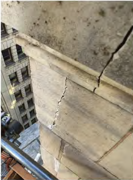
Vertical cracking in historic stone masonry wall assembly resulting from a lack of movement joints to allow for differential settlement and thermal expansion.
