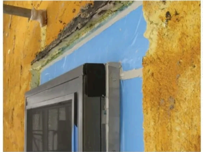
COURTESY: HOFFMANN ARCHITECTS + ENGINEERS
