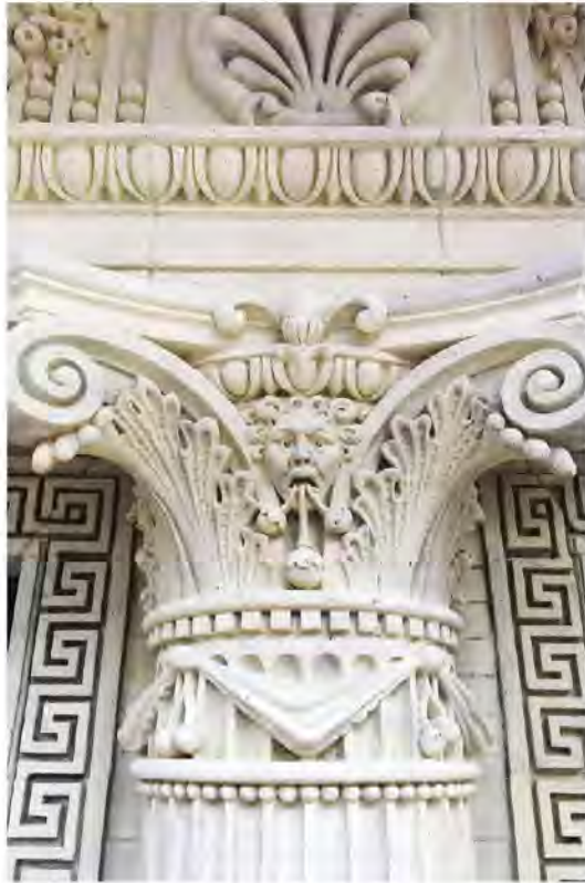
The coating on this decorative terra cotta element protects the surface from exposure. (Similarly, the terra cotta restoration for the midtown Manhattan building shown on page 17 included coating replacement.)
