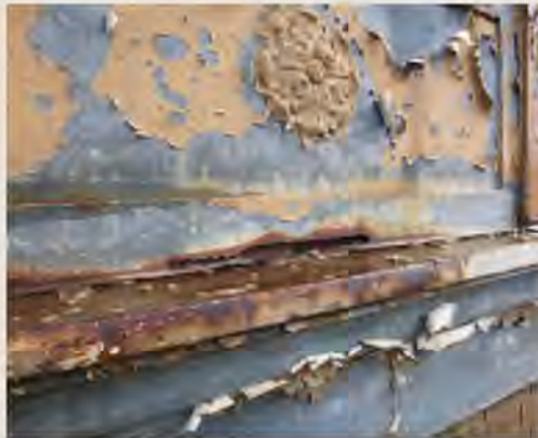
Peeling paint at a decorative metal element.
