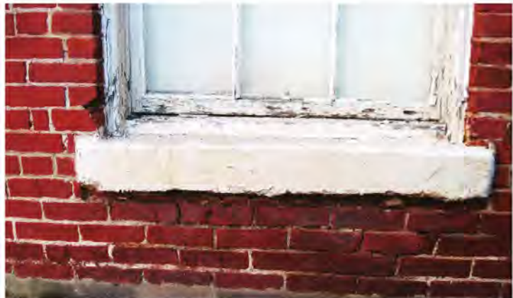
An example of wood window coating deterioration.
