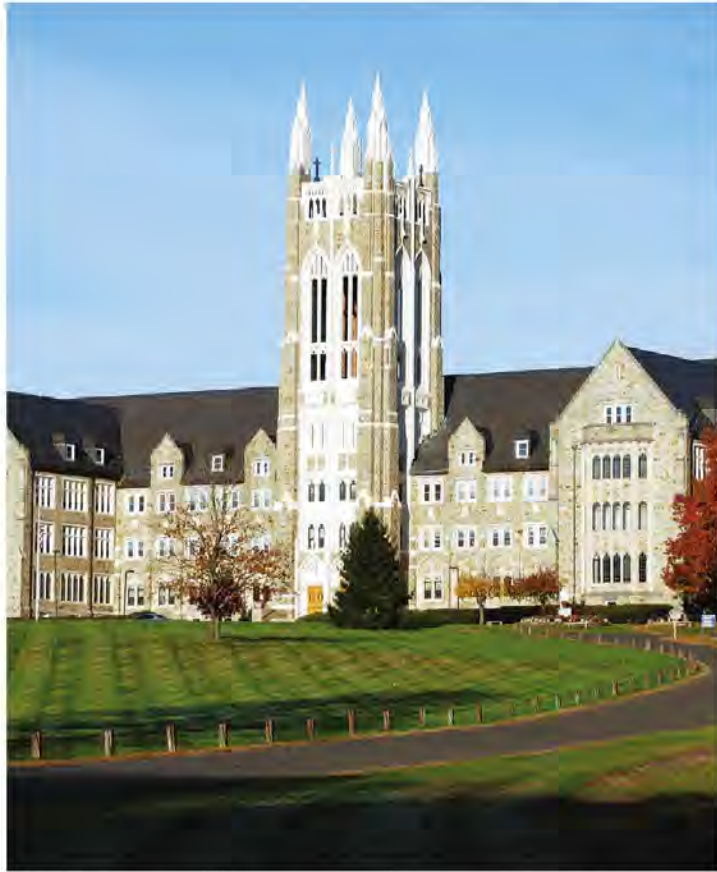
Façade rehabilitation, including limestone coating replacement, restored the bell tower at this historic seminary.
