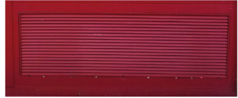
The packaged terminal air conditioning (PTAC) louver, on the exterior face of the wall sleeve, integrated part of the window-wall system. The weep holes were over-drilled at the louver frame, creating an opening between the louver and the window frames.
