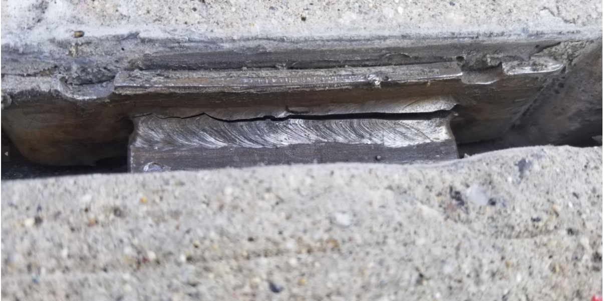
Photo 1 Fatigue failure of weld. Straight, flat weld fracture through throat of weld.
