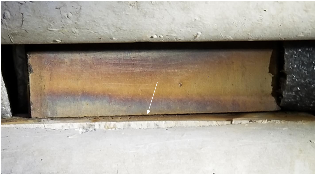
Photo 4 Typical gap between bottom of erection bar and embedment.
