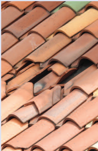
Broken tiles or shingles.
