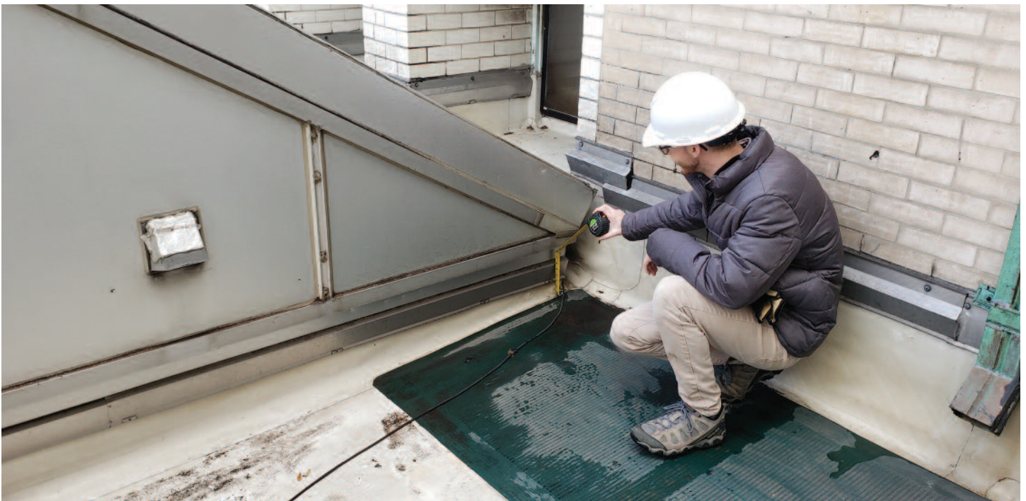
Unless roof surveys are conducted routinely, deterioration can go undetected and lead to premature roofing failure.
