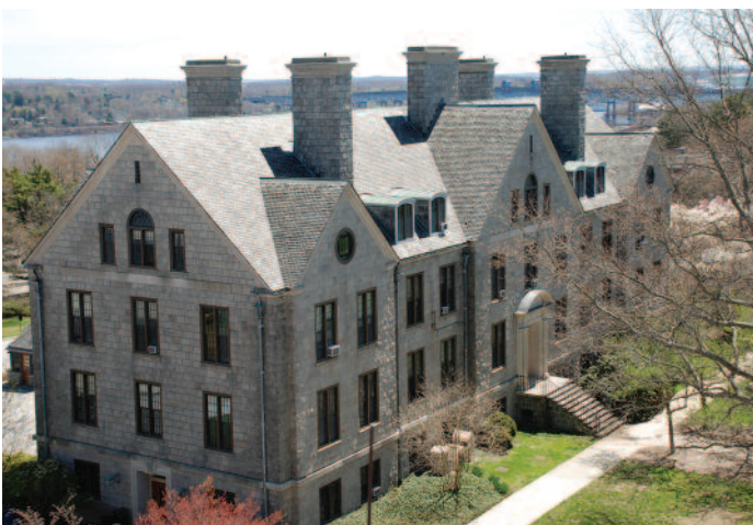
A slate-roof condition survey helped extend the lifespan of the roofing at this historical university hall in New England.
