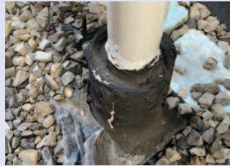
Damage at roof penetrations.
