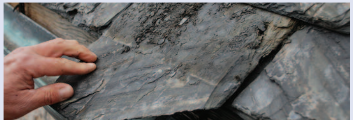
Loose, displaced, or missing shingles.
