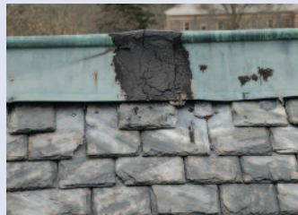
Failed past repairs.
