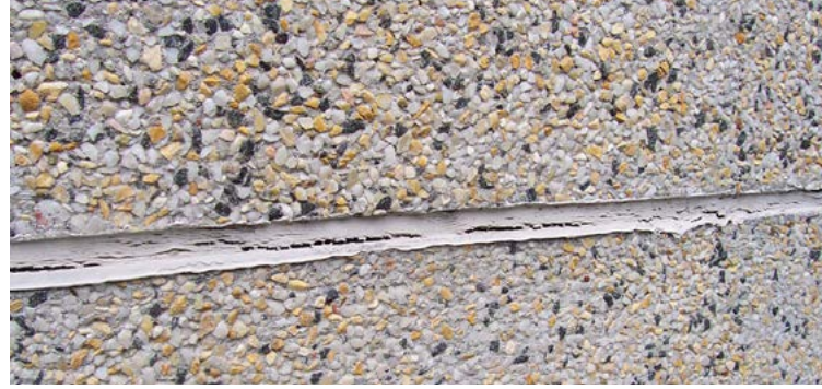
This is an example of cohesive failure where the sealant tears within itself.
