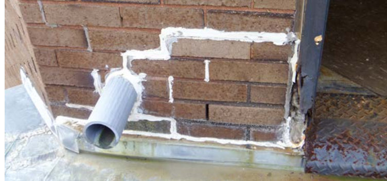
A sealant is being misused to repair mortar joints in this building.
