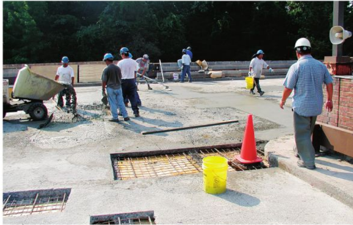
A team carries out the rehabilitation of corroded reinforcement and damaged concrete at a multi-story parking facility.
