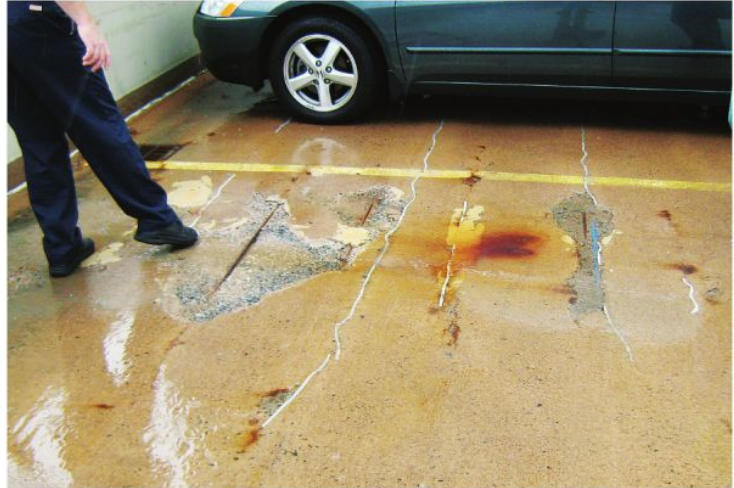
Corrosion of embedded steel reinforcement is a leading cause of premature deterioration in parking garages, like the one shown above.
