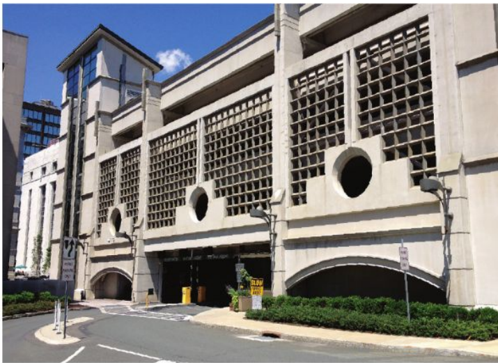
Assessment and repair of this university administration parking garage addressed incipient problems before deterioration could compromise the building's structural and material integrity.
