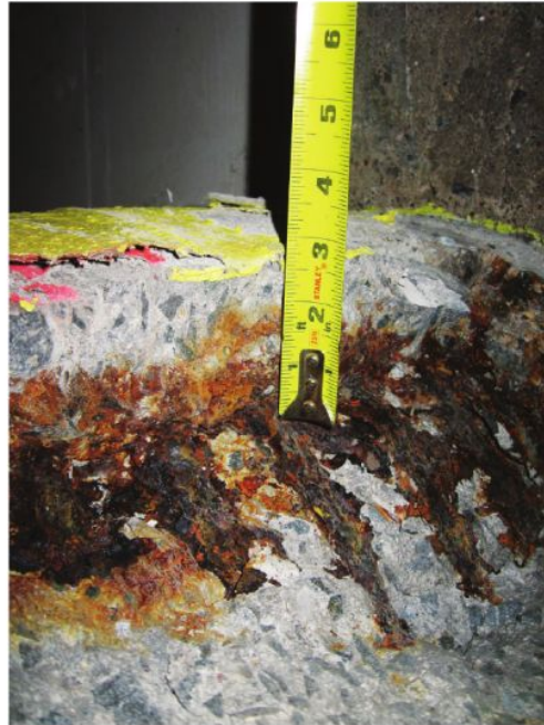
Sufficient concrete cover over reinforcing is essential in order to protect embedded steel from water and dissolved chlorides.
