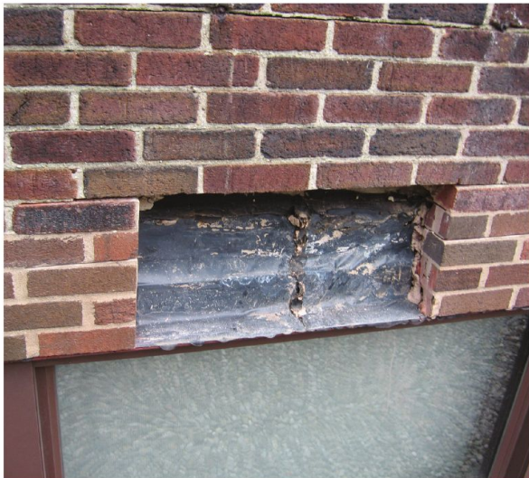
An example of damaged flashing at window head.
