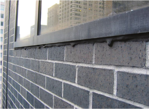
Sealant failure at the exterior of a window.
