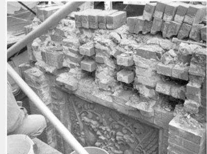
▲ Severely deteriorated brick at the hotel necessitated complete reconstruction of the upper exterior walls and replacement of face brick at lower areas.
